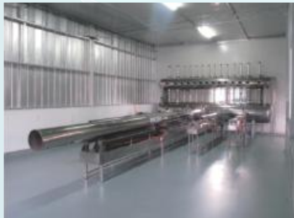
Gas Flow Calibration Station (Size: DN15–DN300)
